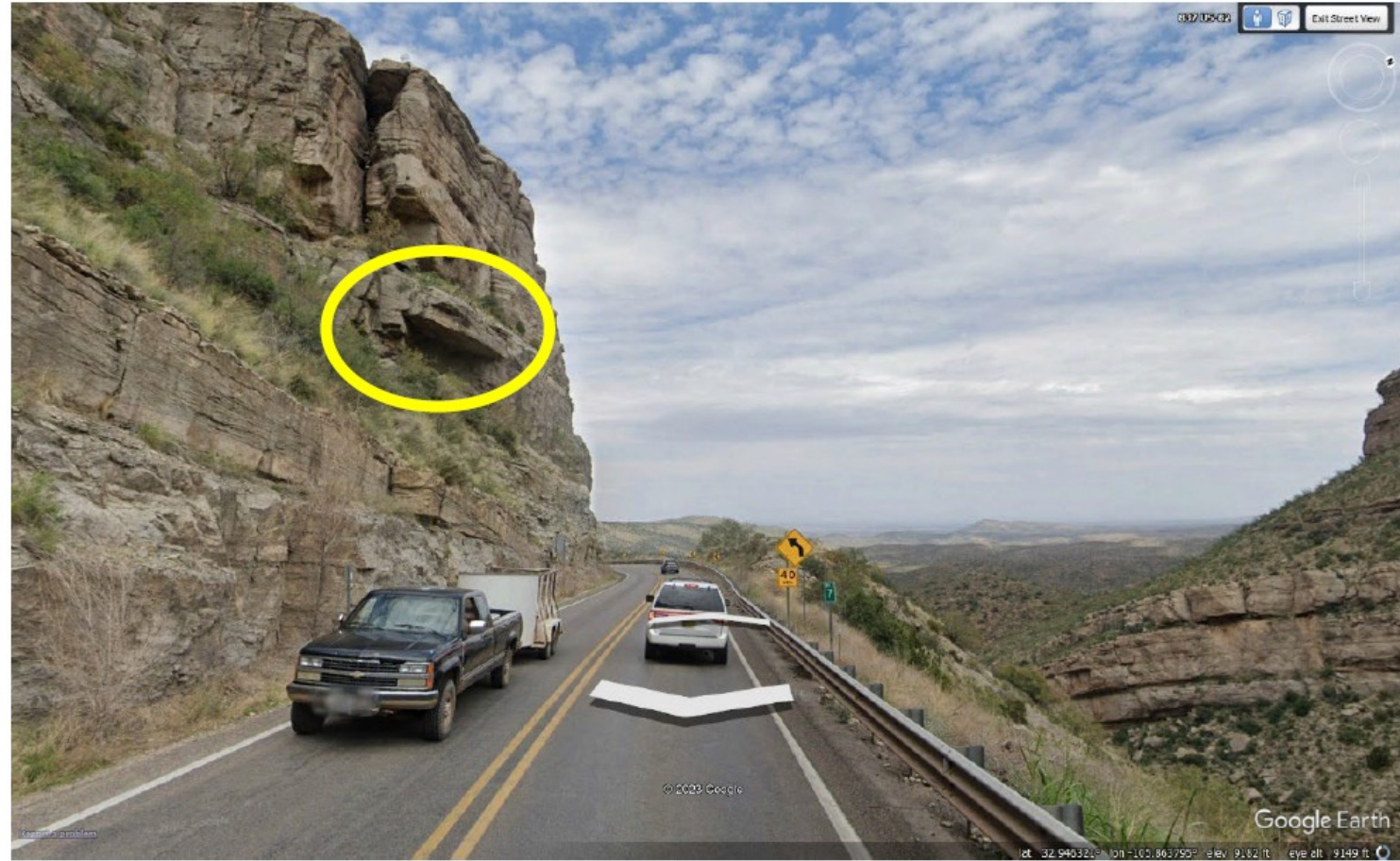
Figure 1: Pre-failure screen capture from Google Street View. Dislodged limestone block circled in yellow.
