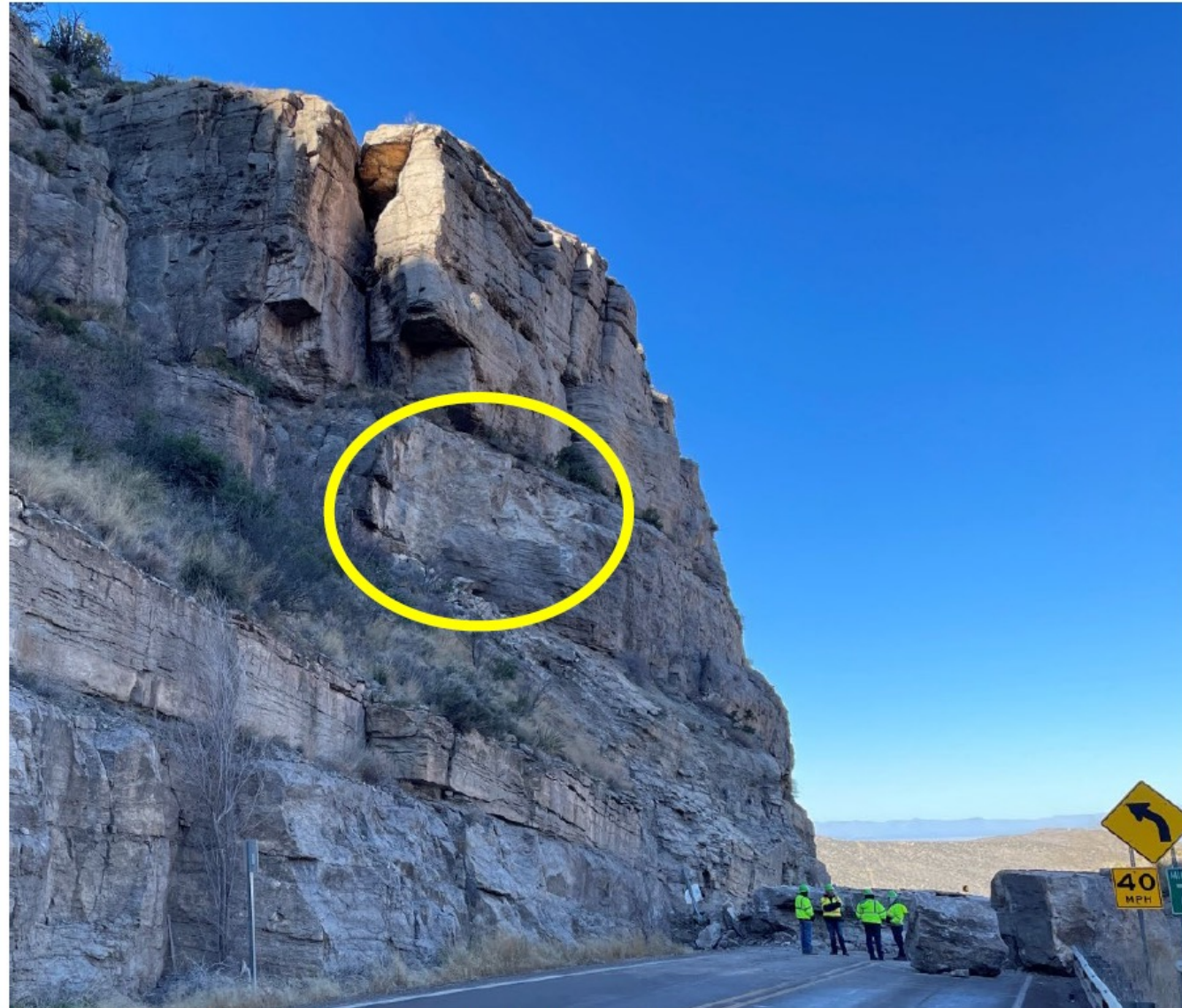
Figure 2: Post-failure photo. Rockfall scarp circled in yellow.
