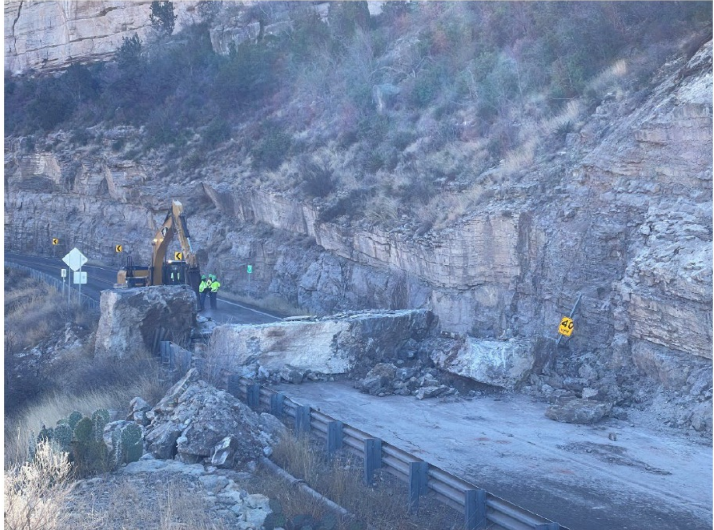
Figure 3: Overview photo of rockfall prior to cleanup of largest blocks.
