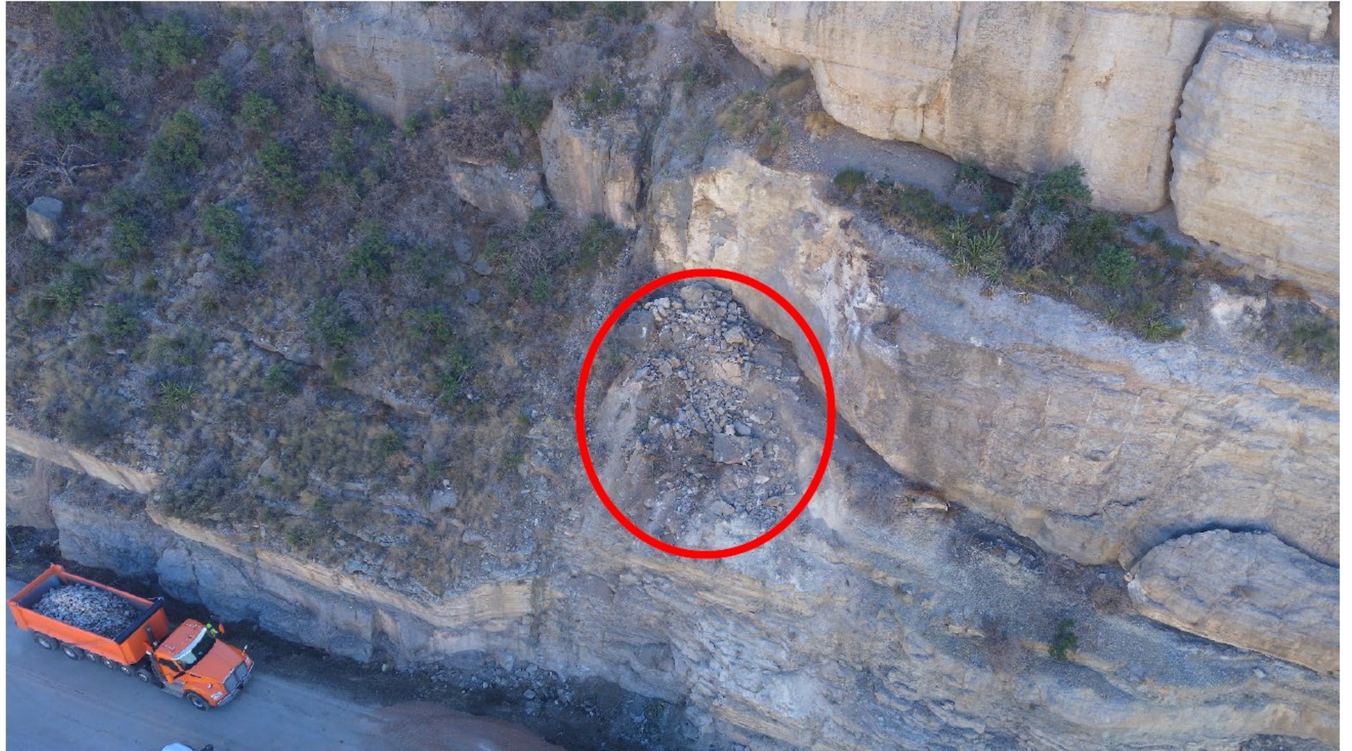
Figure 4: Leftover rockfall debris on the slope, circled in red. Recommended to clean up by scalers or future storm events could bring this material to the roadway below. Temporary concrete barrier below this area should be considered until scaling can be performed.
